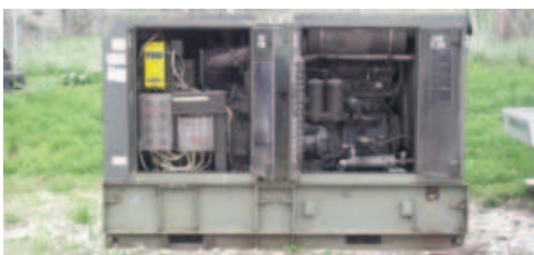
200 KW Generator Set MFG: Freemont Bridgeport SN:VZ00573 $10,000.00
