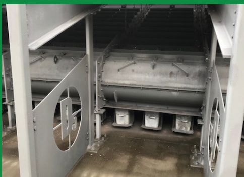
The rounded "drum" section is a deceleration chamber that slows the projectiles before they are dropped into the buckets below
