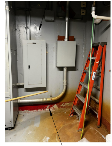
A SCRAPE FLAKING PAINT ON WALL SURFACE. CLEAN AND PREPARE FOR NEW PAINT.
