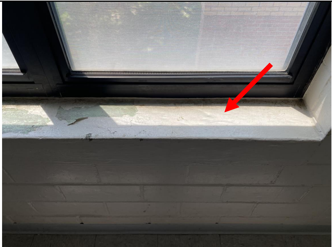
View of windowsill with LBP.
