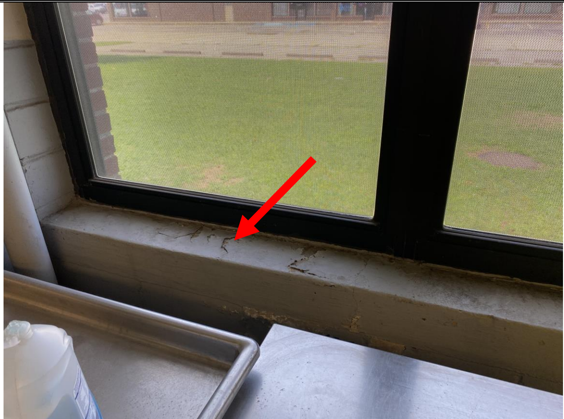
View of windowsill with LBP.
