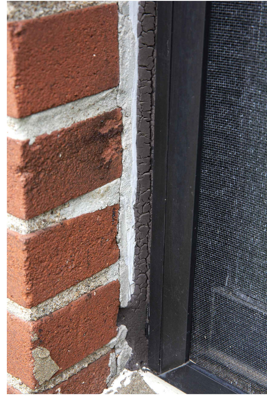
2 EXTERIOR SEALANT DETERIORATION NTS
