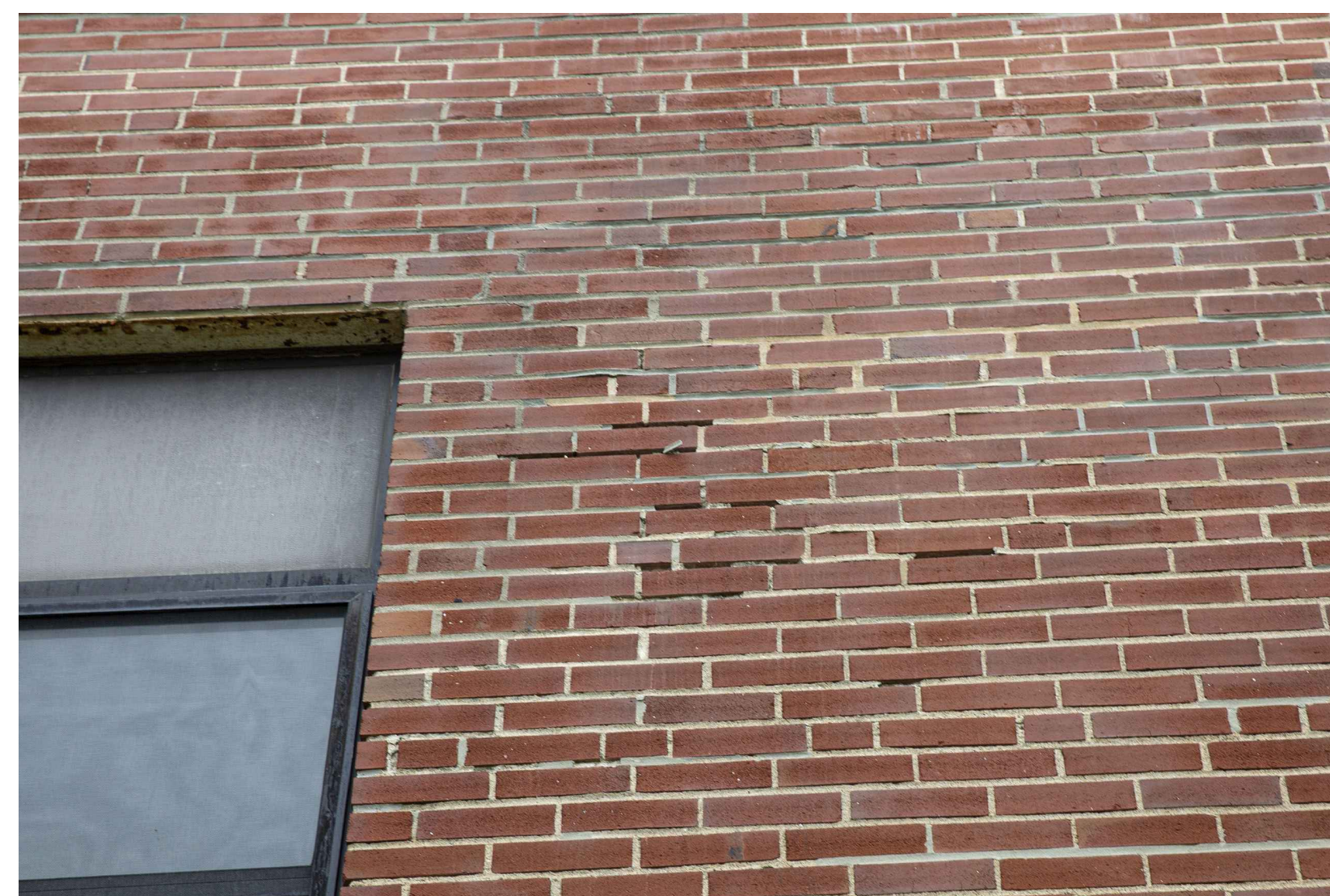
8 EXTERIOR MORTAR DAMAGE NTS
