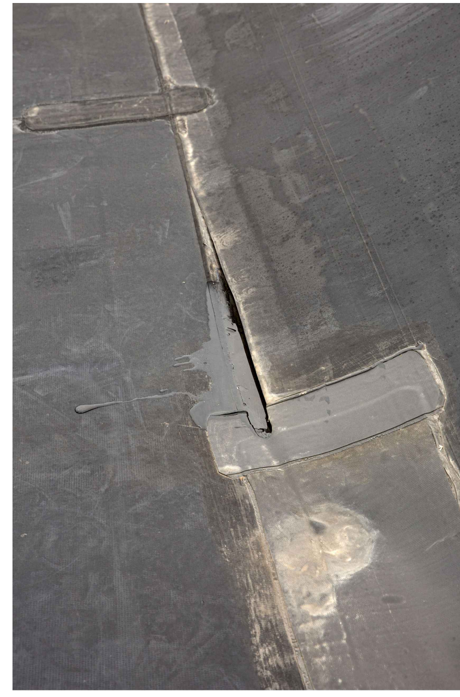
3 ROOF DAMAGE NTS
