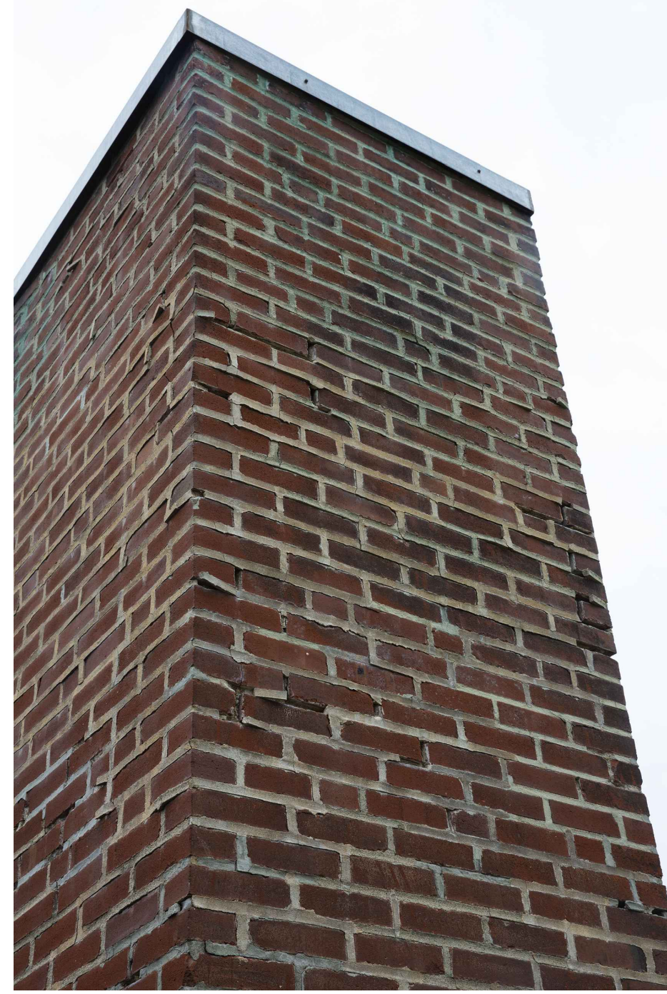
1 EXTERIOR MORTAR DAMAGE NTS
