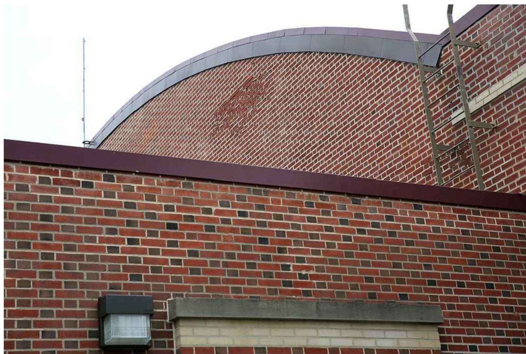
5 EXTERIOR MORTAR DAMAGE NTS
