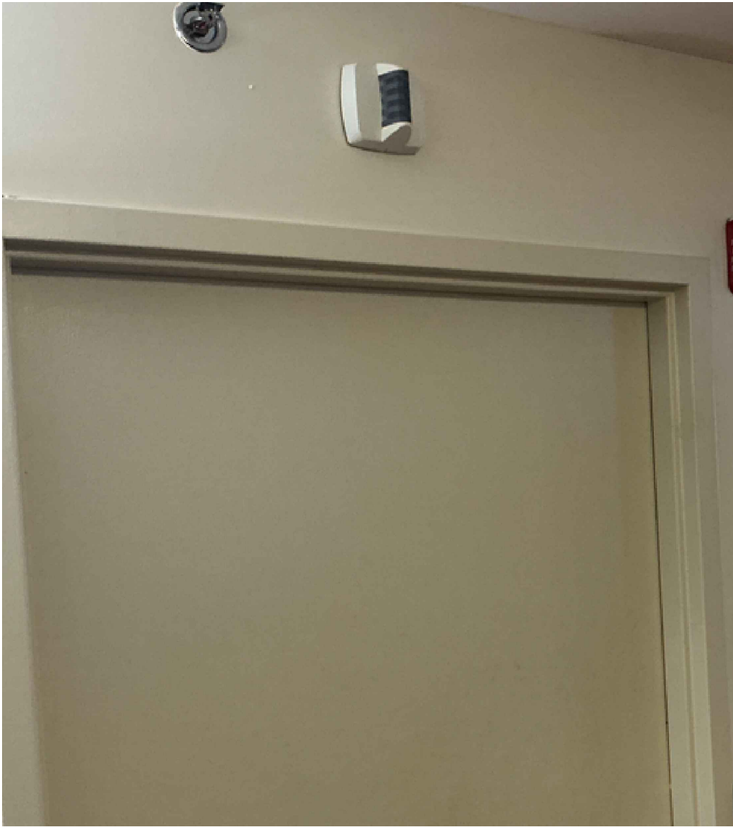
TYPICAL CURRENT DOME LIGHT, SOME LOCATIONS ARE CEILING MOUNTED
