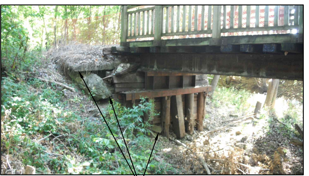
SITE PHOTO 2 NOT TO SCALE RELOCATE EXISTING CONCRETE RUBBLE SHOWN TO BE ON LEFT SIDE OF EMBANKMENT FROM STATION 11+50 TO 12+00
