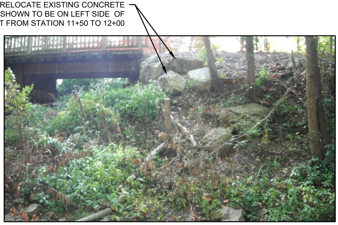
SITE PHOTO 5 NOT TO SCALE RELOCATE EXISTING CONCRETE RUBBLE SHOWN TO BE ON LEFT SIDE OF EMBANKMENT FROM STATION 11+50 TO 12+00
