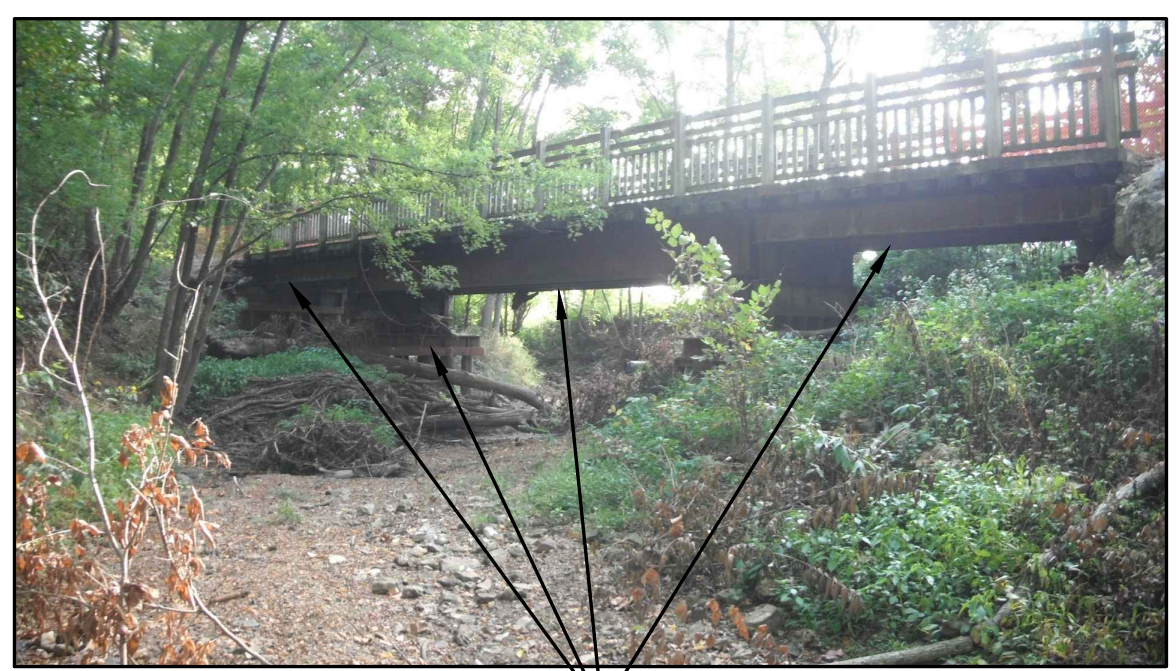
SITE PHOTO 1 NOT TO SCALE REMOVE ENTIRE EXISTING 3-SPAN BRIDGE WITH STEEL & TIMBER FRAMING FROM SITE
