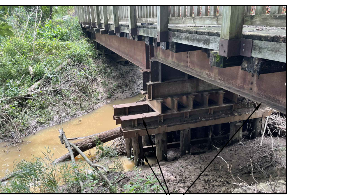
SITE PHOTO 3 NOT TO SCALE REMOVE ENTIRE EXISTING 3-SPAN BRIDGE WITH STEEL & TIMBER FRAMING FROM SITE
