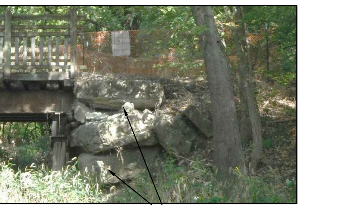
SITE PHOTO 4 NOT TO SCALE RELOCATE EXISTING CONCRETE RUBBLE SHOWN TO BE ON LEFT SIDE OF EMBANKMENT FROM STATION 11+50 TO 12+00
