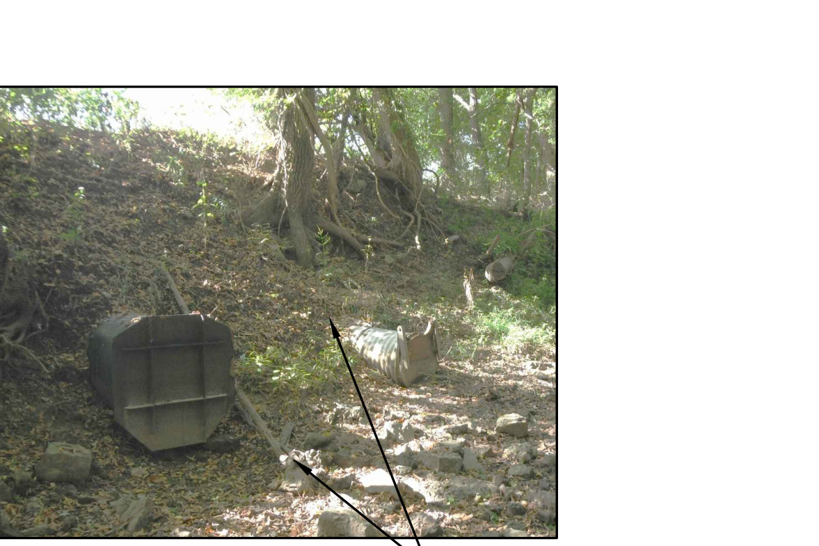
SITE PHOTO 7 NOT TO SCALE DO NOT DISTURB EXISTING CMP PIPE FLOOD CONTROL STRUCTURES
