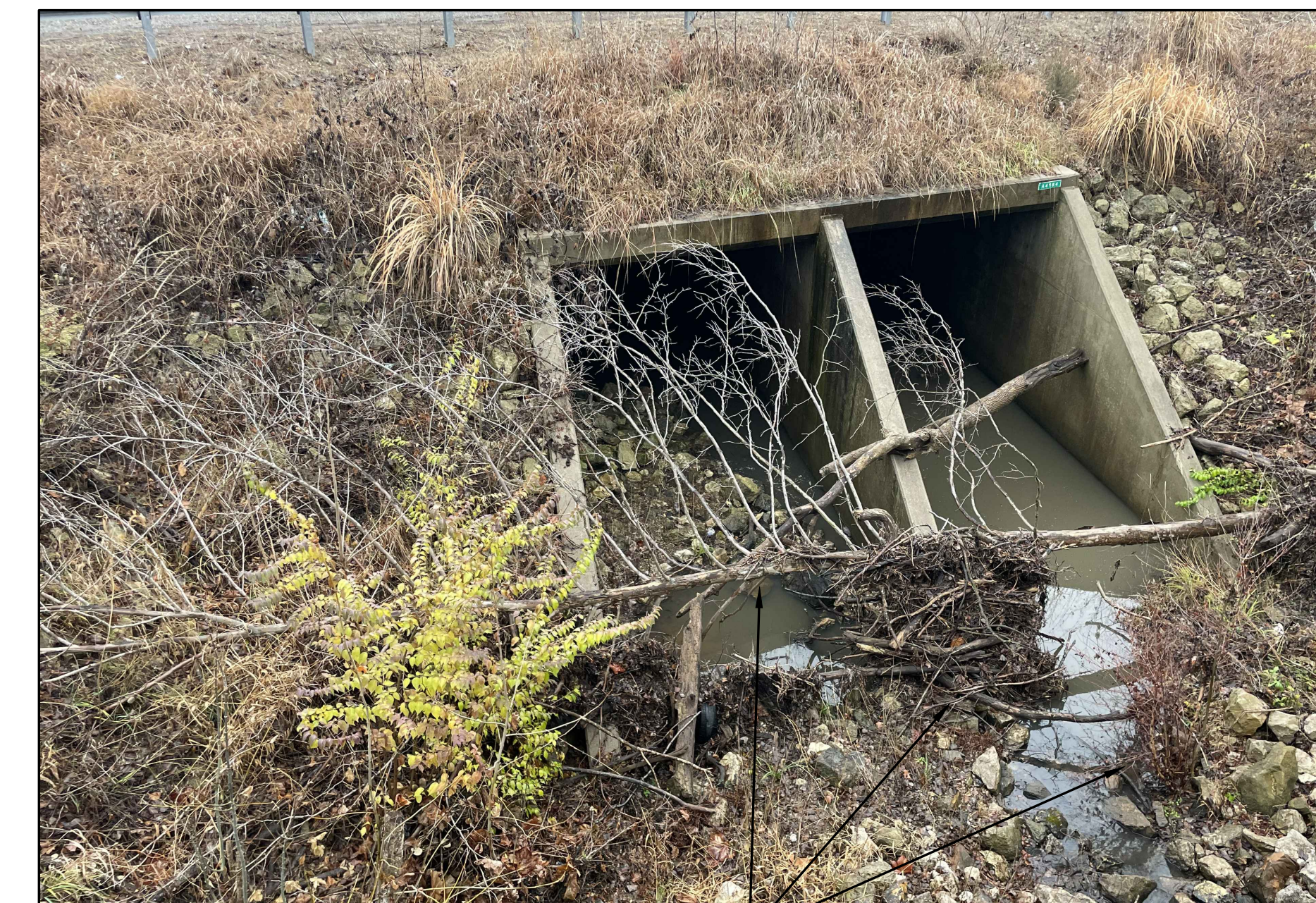
REMOVE ALL DEBRIS FROM BOX CULVERT OPENING INCLUDING CLEARING AND GRUBBING VEGETATION WITHIN BOTTOM OF STREAM BANKS SITE PHOTO 3 NOT TO SCALE
