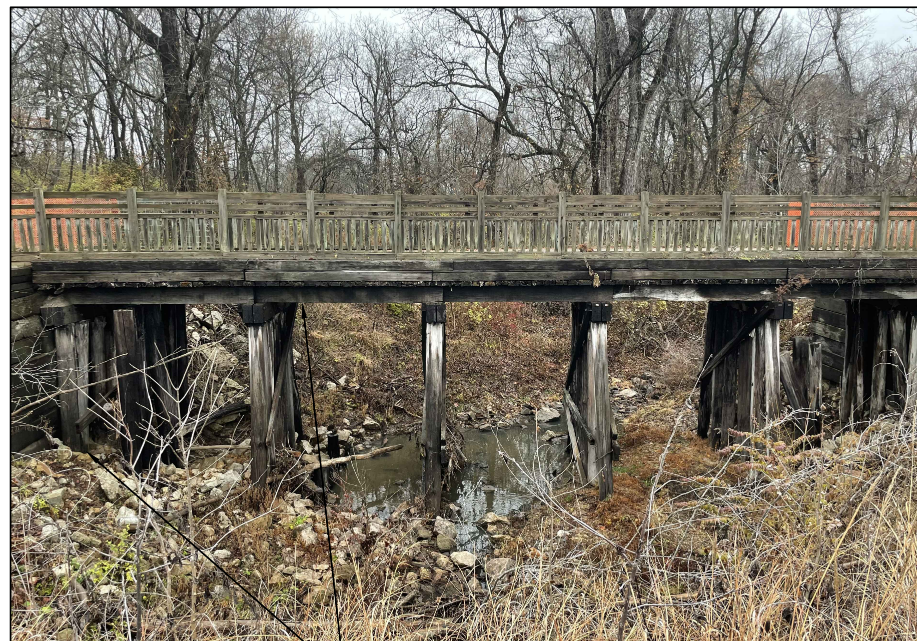
REMOVE ENTIRE EXISTING 6-SPAN BRIDGE WITH TIMBER FRAMING AND END BENTS FROM SITE SITE PHOTO 1 NOT TO SCALE
