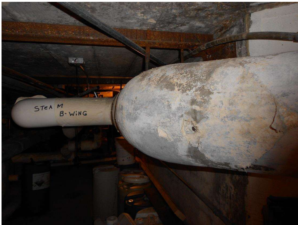
Figure 2: Bldg. 3, B-Wing steam line in tunnel
