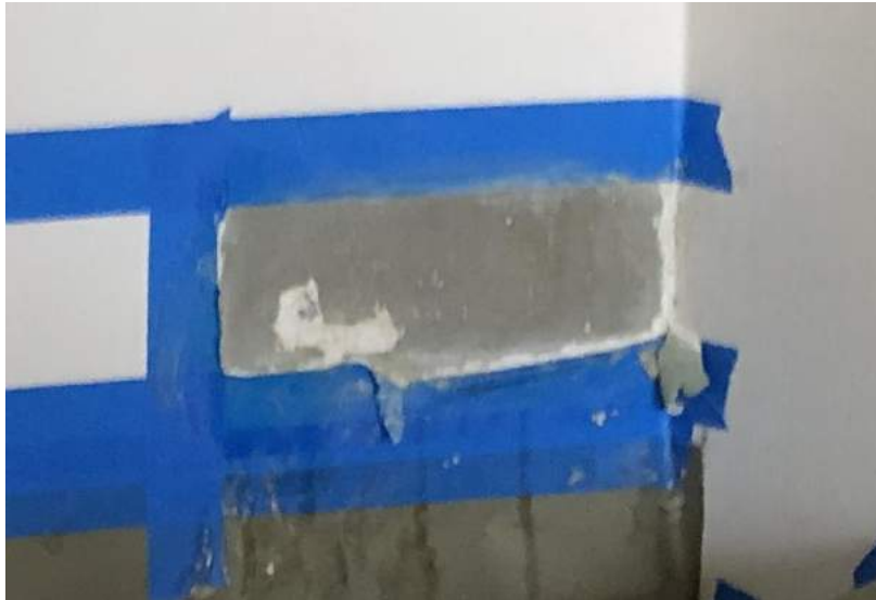
Exposure at the walls.
