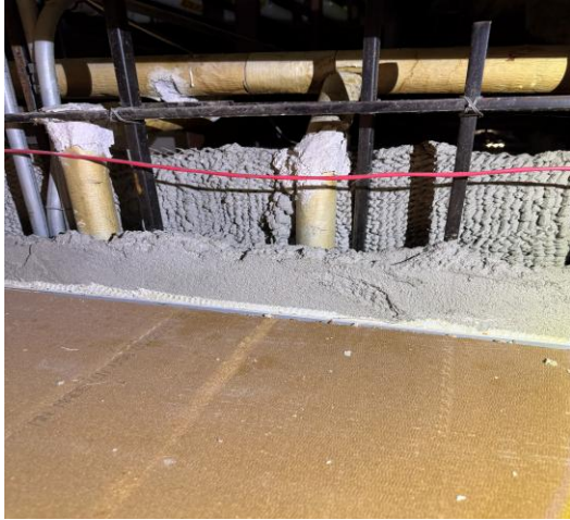
Basement Restroom line Museum
