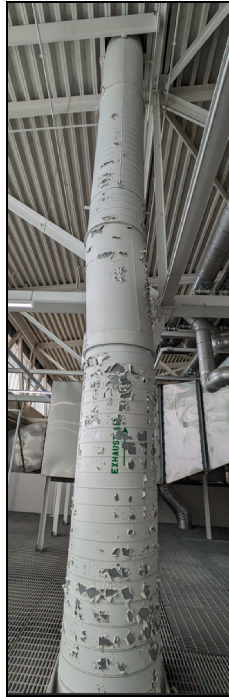
EXHAUST AIR COLUMN
