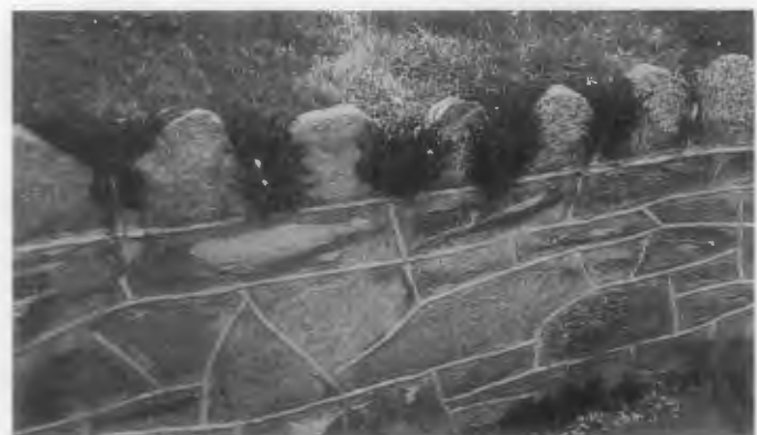
Figure 20. This stone garden wall was tuckpointed to match the tuckpointing on the c. 1920s house on the property. Photo: Anne Grimmer.
