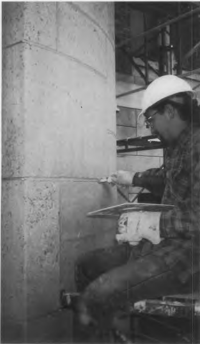
Figure 1. After removing deteriorated mortar, an experienced mason repoints a portion of this early-20th century limestone building. Photo: Robert C. Mack, FAIA.
