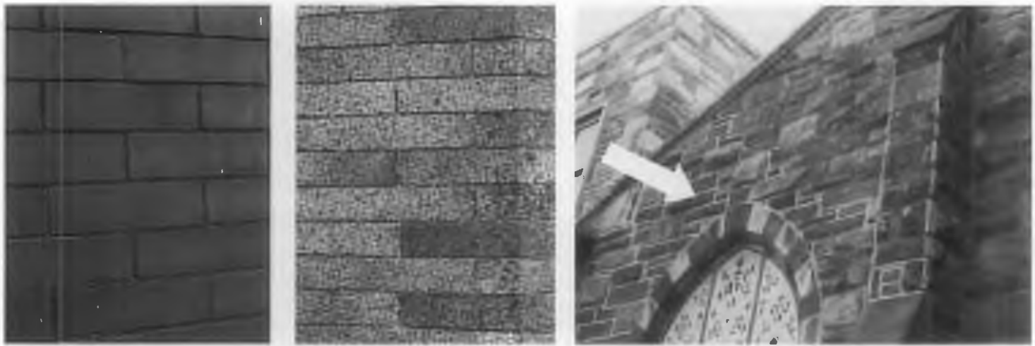
Figure 6. Tinted mortar. (left) Black mortar with a beaded joint was used here on this late-19th century hard pressed red brick and, (center) a dark brown tinted mortar with an almost flush joint was used on this early-20th century Roman brick. (right) When constructed at the turn-of-the-century, this building was pointed with a dark gray mortar to blend with the color of the stone, but the light-colored mortar used in spot repointing has destroyed this harmony and adversely impacts the building's historic character. Photos: Anne Grimmer.
