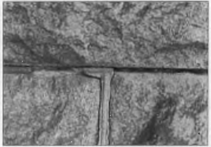
Figure 8. Due to inadequate joint preparation, the repointing mortar has not adhered properly and is falling out of the joint. Photo: Robert C. Mack, FAIA.
