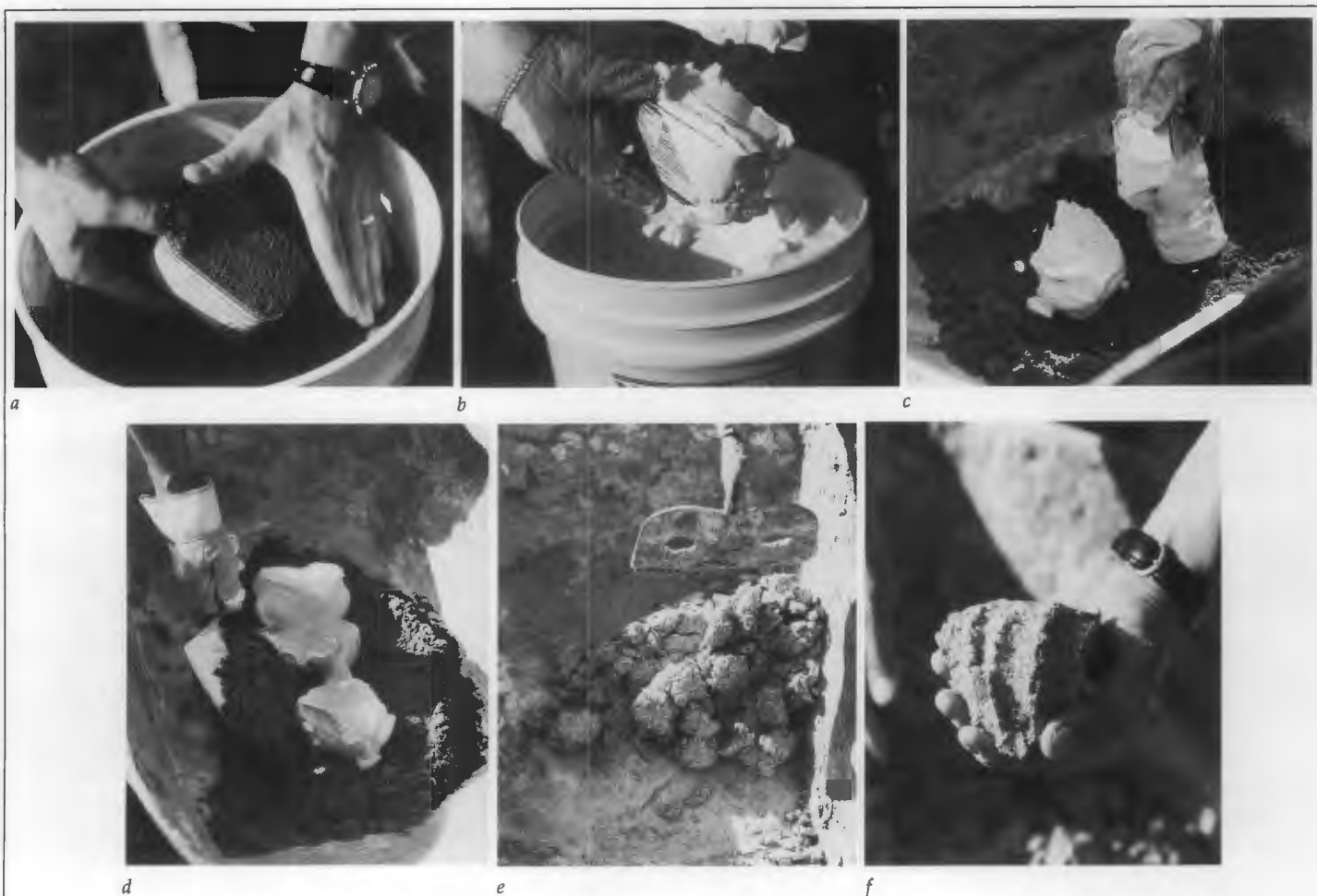
Figure 14. Mixing mortar using lime putty: (a) proportioning sand; (b) proportioning lime putty; (c) placing lime putty on top of sand; (d) mixing sand over lime putty; (e) hand mixing mortar; and, (f) sample of mortar after mixing. Photos: John P. Speweik.
