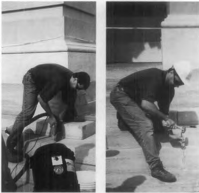
Figure 13. (left) In preparation for repointing, the mortar joints on these granite steps are first cut out mechanically (note the vacuum attached to the cutting tool in foreground to cut down on dust). (right) Final removal of the old mortar is done by hand to avoid damage to the edges of the joints. Mechanical preparation of horizontal joints by an experienced mason may sometimes be acceptable, especially where the joints are quite wide and the masonry is a very hard stone. Photos: Anne Grimmer.
