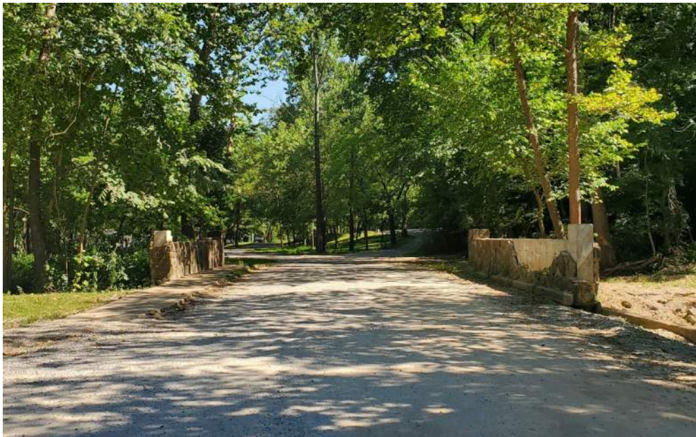
Figure 9: Bridge 4 – Looking west at deck and roadway, missing stone veneer on each barrier
